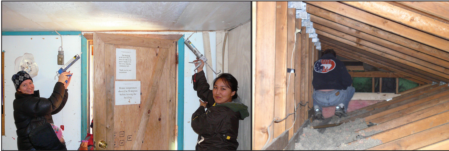
Left: Caulking the Nightmute Community Hall. Right: Insulation being installed into a roof space of a residence in Fairbanks.
